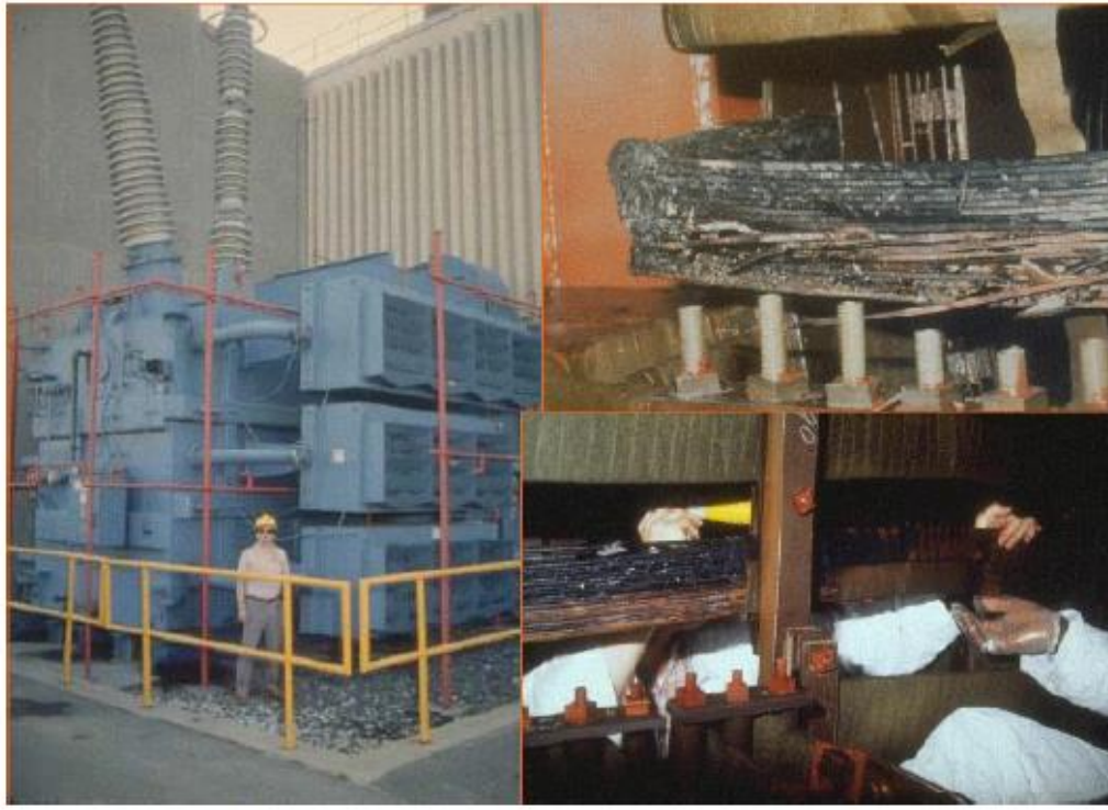
March 1989 magnetic storm damage to a high-voltage transformer at a nuclear power center in Salem, New Jersey.
