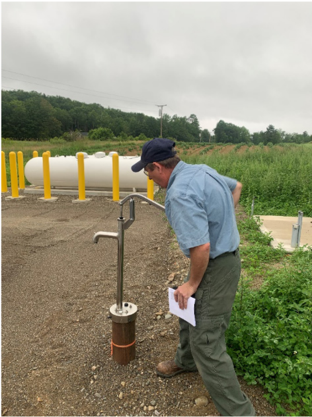
Figure 5. Waldo EMA Director Dale Rowley demonstrates the manual pump capability for the EOC's well. In background can be seen the three 1000-gallon propane tanks that provide off-grid heat and back-up power generation capability.
