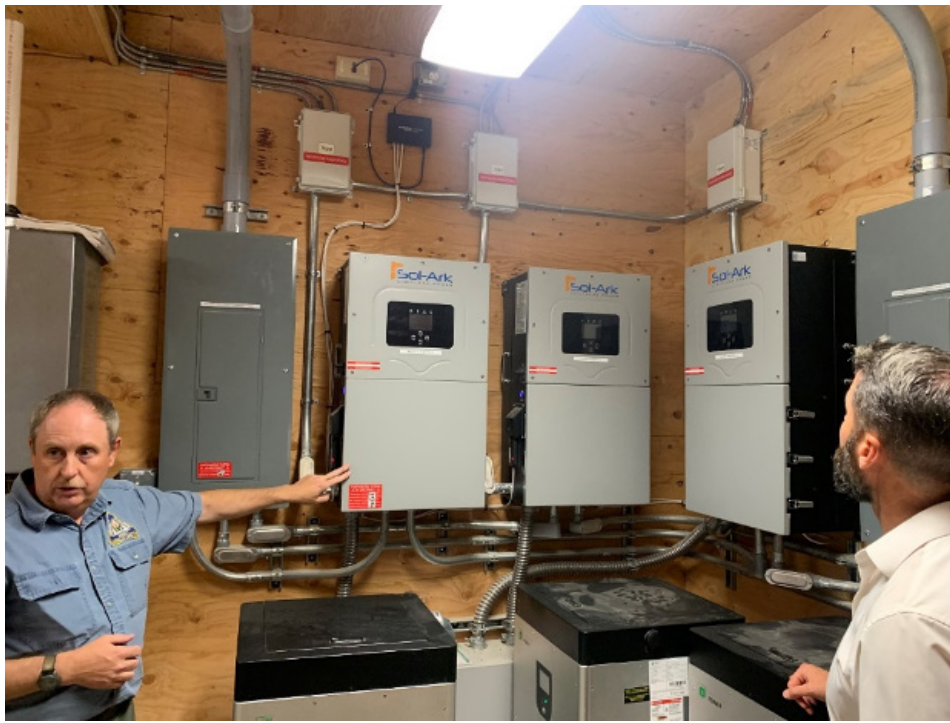
Figure 2. Director Dale Rowley shows CSP president Tommy Waller the operation center’s Sol-Ark inverters. These inverters provide the EOC with sufficient power, and actually reduce the county’s monthly energy bill while helping to provide off-grid capability.
