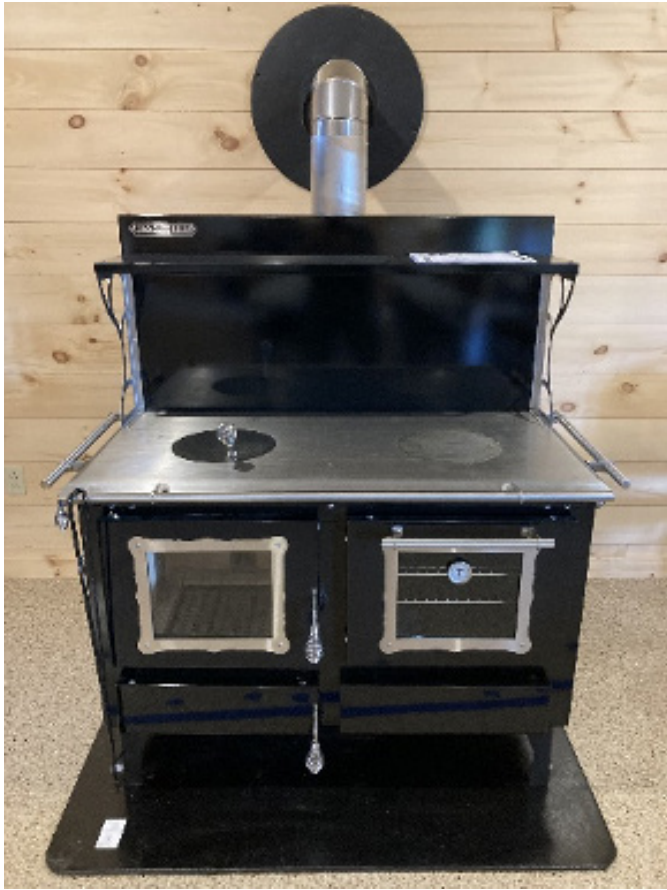
Figure 3. Amish-built wood-fired cookstove provides secondary heating and cooking capability. Many Maine houses utilize wood stoves for supplemental heating during the state's long winters.
