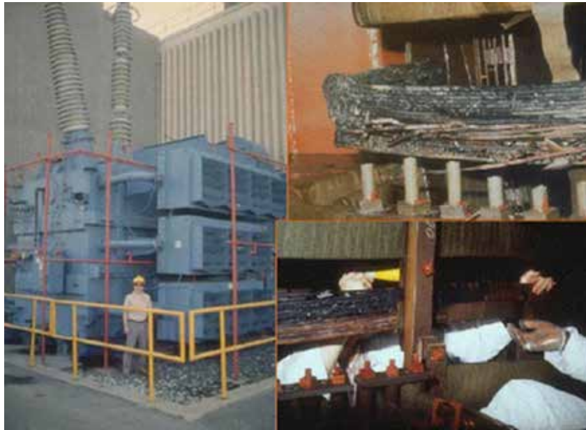
March 1989 magnetic storm damage to a high-voltage transformer at a nuclear power center in Salem, New Jersey. Photo credit: Dr. Jeffrey J. Love, USGS
